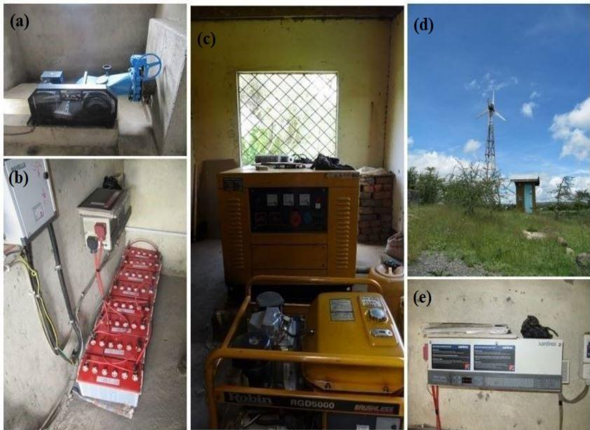
Figure 4: Energy sources at Ngarenanyuki school before deployment of E4G project: (a). a 3.2 kW run-off-river micro-hydropower (MHP) plant, Banki type, (b) Inverter-based PV DC backup systems of 940 W coupled with 1400 Ah/12V battery bank, (c) 5 kW diesel generator, (d) non-operational wind turbine, (e) Inverter
