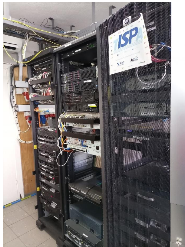
Figure 1: Real application cluster (RAC) of server room
