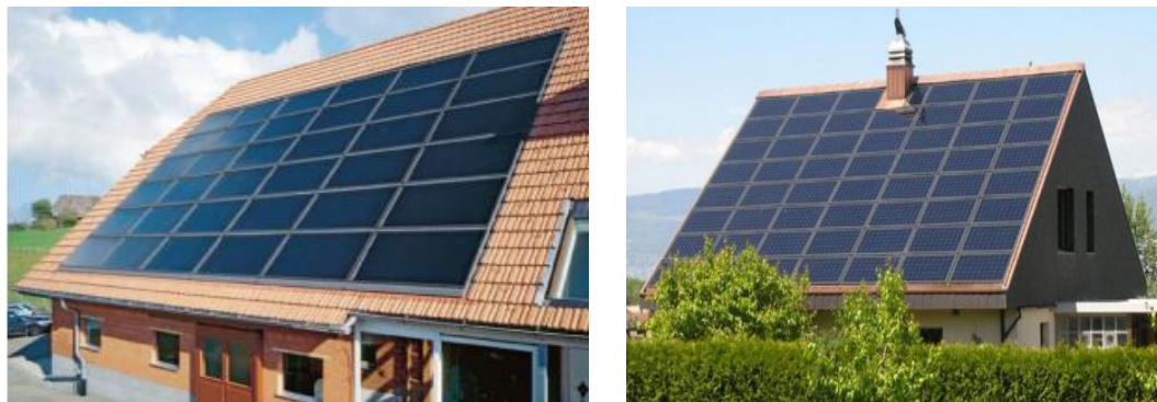
Figure 3: BIPV installation: Framed in-roof system: Less homogenous appeal is due to the contrast of the aluminum frame and PV panels (Skaaland, Ricke, Wallevik & Strandberg, 2011).
