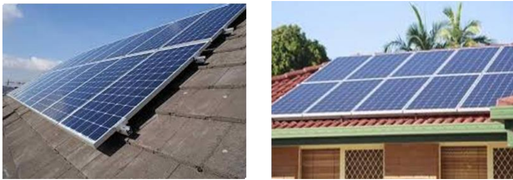
Figure 2: Projects installation with building-applied PV in Tanzania.
