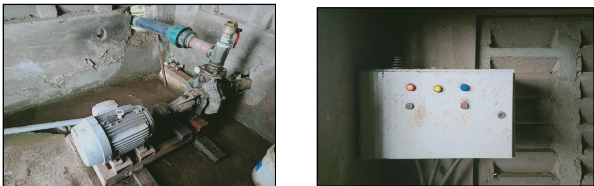
Figure 3: Manual water pump (left) and manual switch-box (right)
