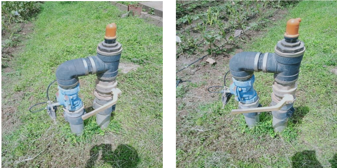
Figure 4: Manual gate valves
