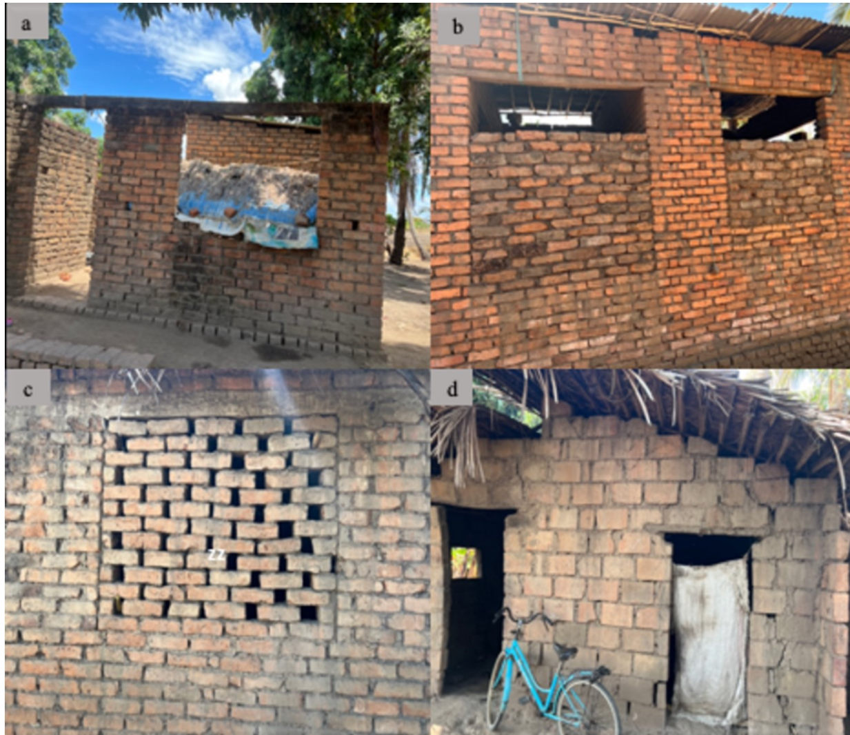
Figure 8: Examples of improved but incomplete houses that people were residing in: (a) un-roofed house, (b) bricks on windows with small gaps on top, (c) holes on the walls and open eaves and (d) no door or window covers installed
