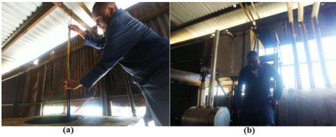
Fig. 1. RABEC Fuel monitoring (a) using a stick and a manual meter (b) descent of the RABEC operator from the top of the fuel tank.
