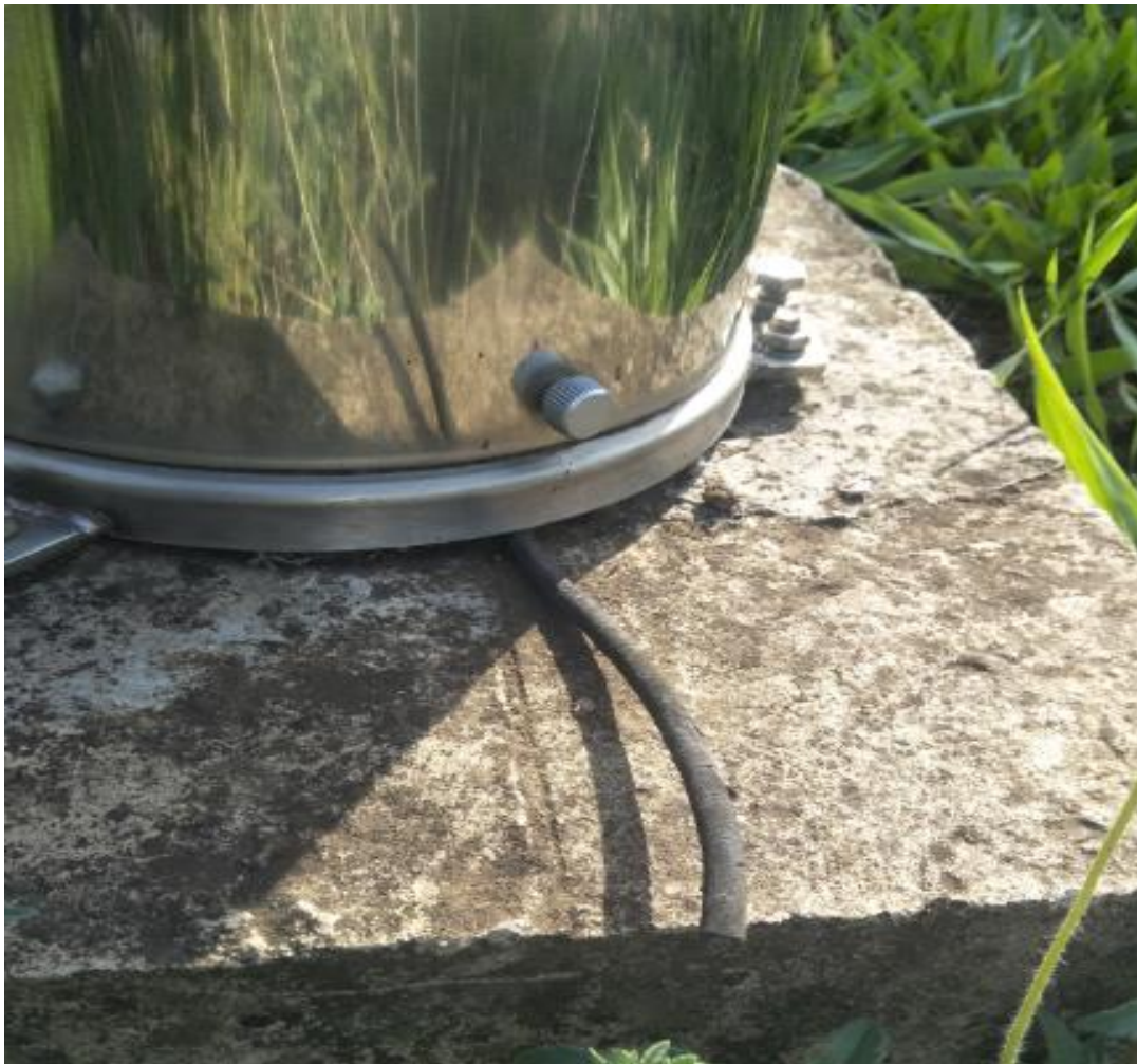
Figure 17: Vandalized rain-gauge which was used in the automatic meteorological station
