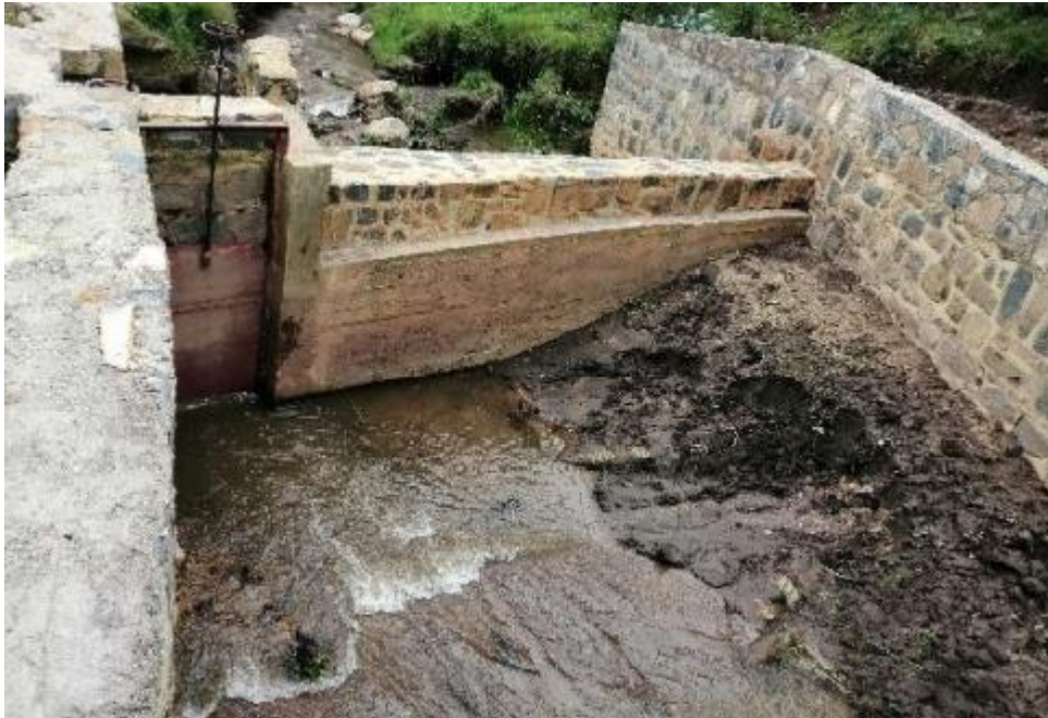
Figure 4: Intake of Mudasomwa pico-hydropower plant (Hobuka Company, 2021)
