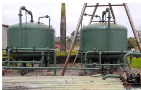
Figure 4 | Activated carbon filters.
