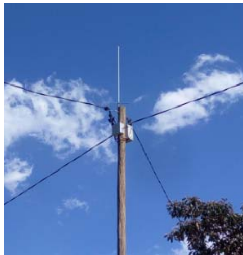
Fig.8. LPWAN Base Station For Enhancing Data Collection
