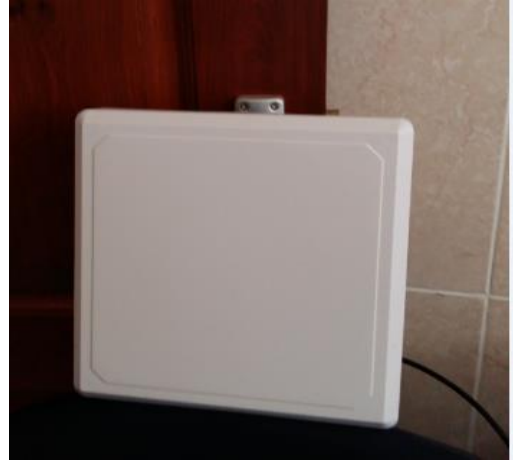
Figure 14: RFID reader antenna place at height of 1m
