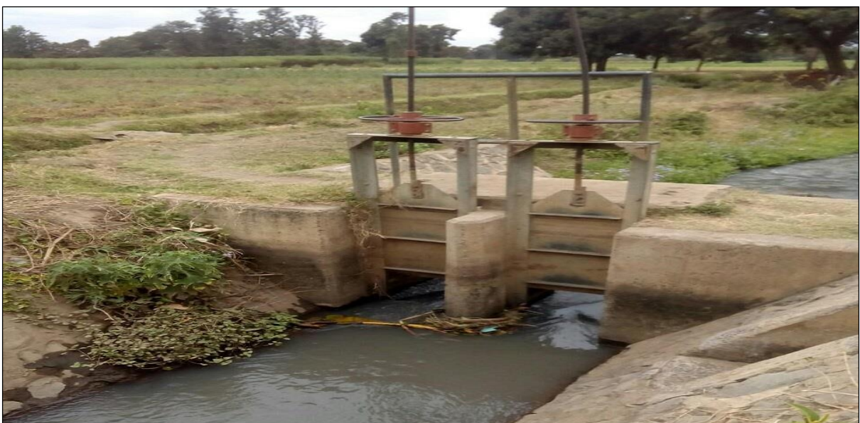
Figure 2: Canal lockable intake gate
