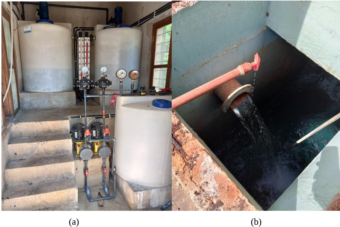
Figure 44: Chlorination plant (a) and water chlorination (b)
