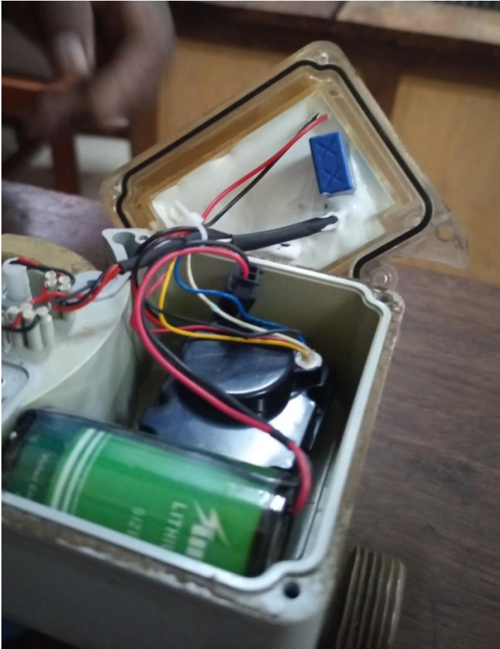
Figure 5: Opening the prepaid meters after removing the top cover
