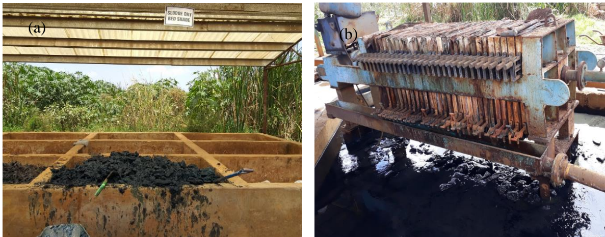
Plate 1: Final Discharge Tank (a) and the Filter Press (b)
