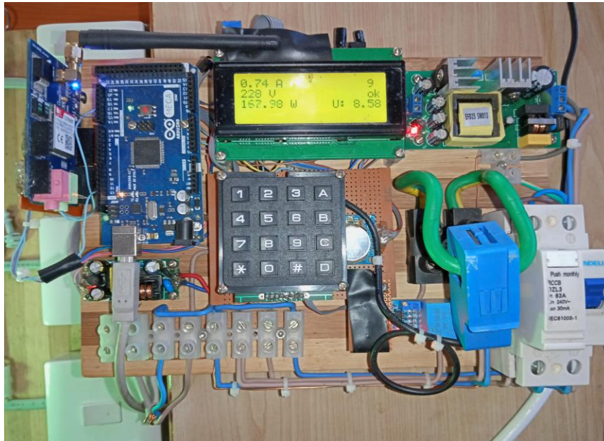
Figure 24: Smart meter unit during system testing
