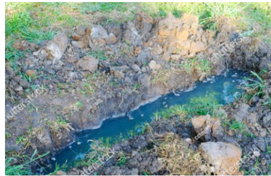
Figure 21: Physical damage of the system with the first-hand release of raw sewage
