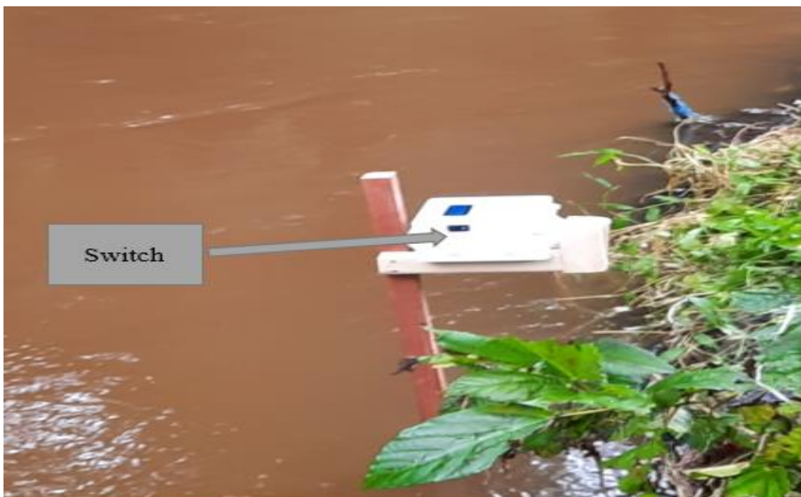
Figure 25: System installed at the field
